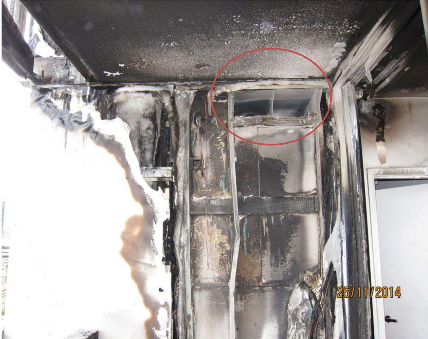
Figure 19 - Apartment Exhaust Duct
