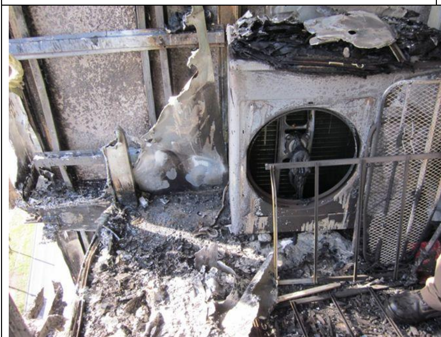
Photo of base of wall and penetrations plus overhang past balcony edge
