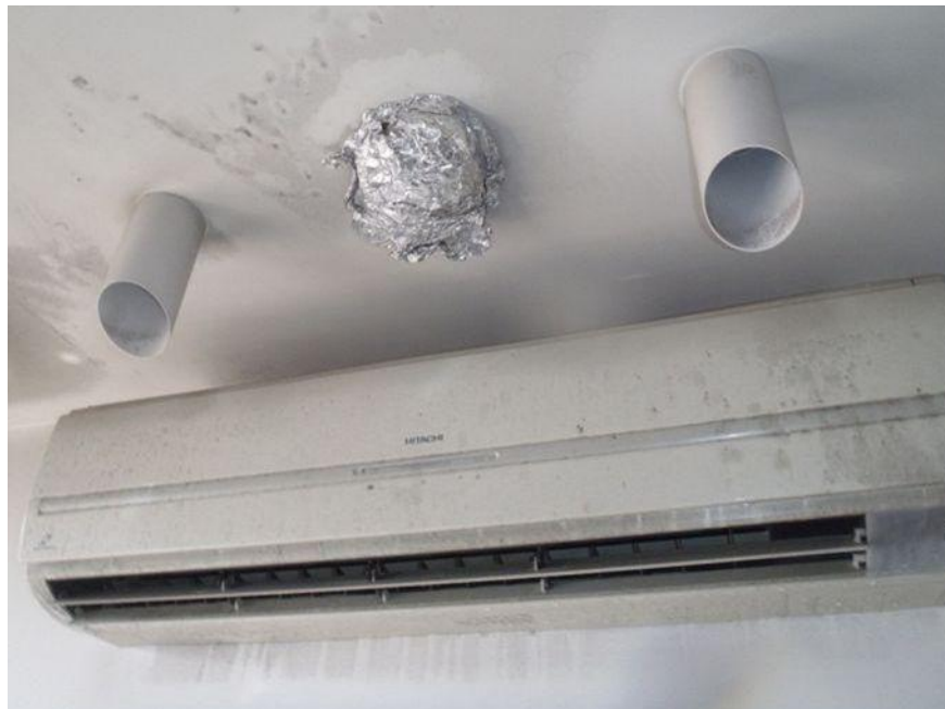
Figure 14 - An example of an obstructed Smoke Alarm – Apartment 805
