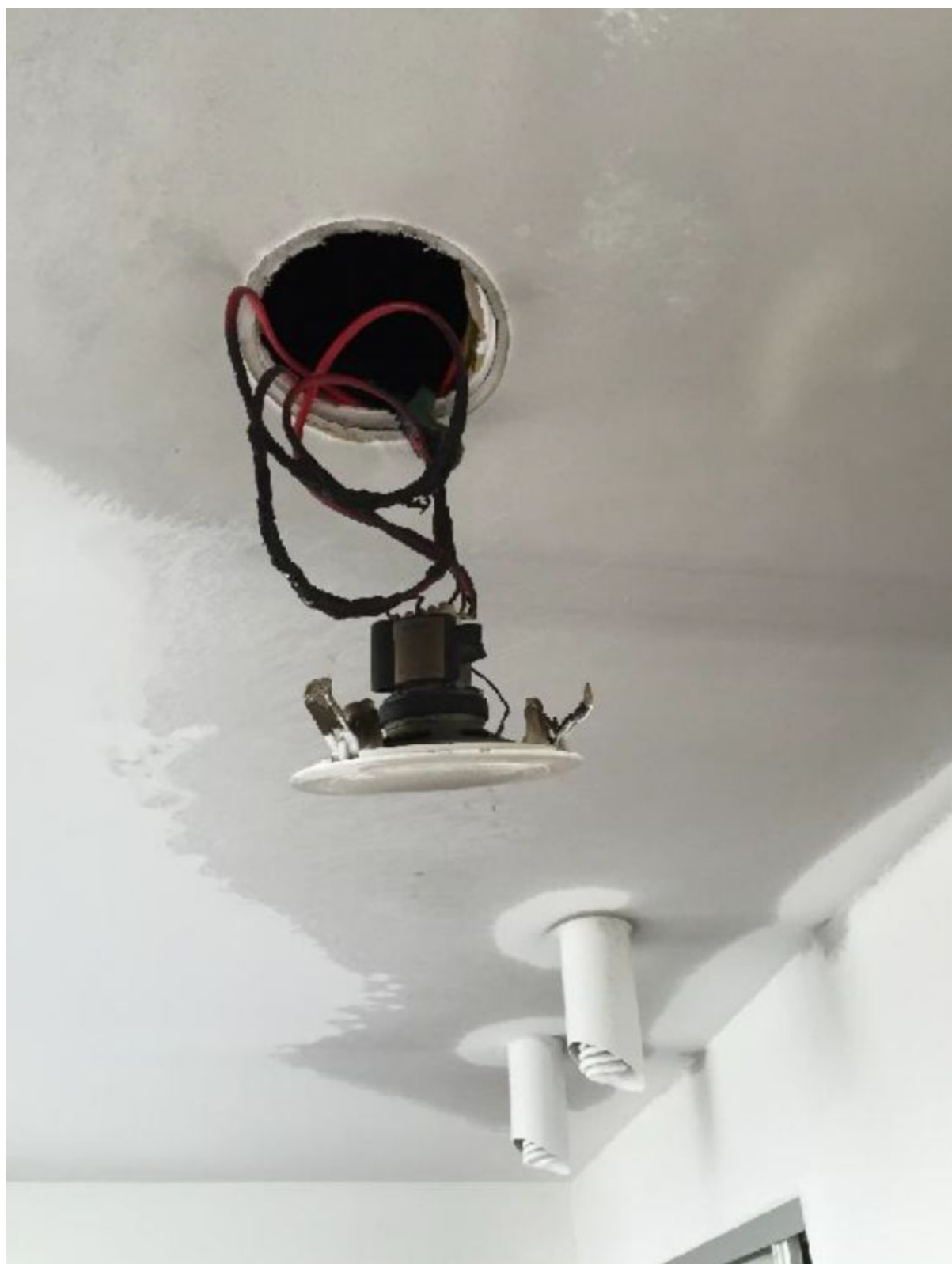
Figure 20 - EWIS Speaker and wiring
