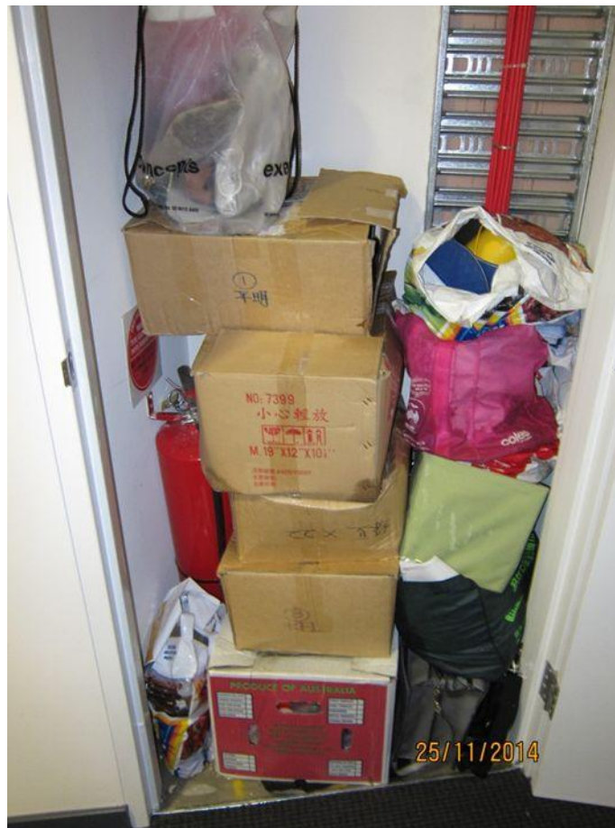
Figure 13 - Fire extinguisher cupboard on Level 6.
